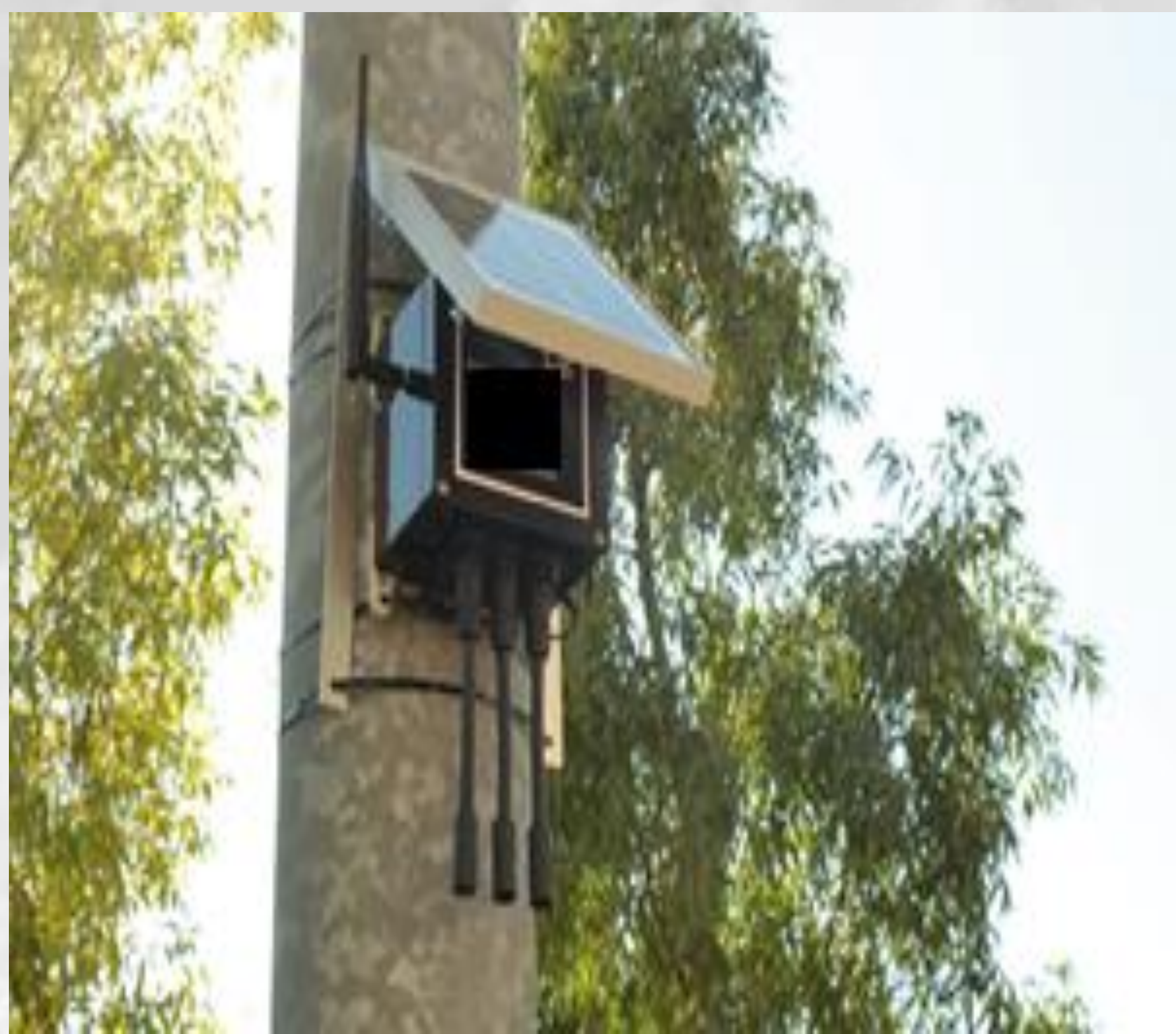
Air quality monitoring station powered by an external solar panel
